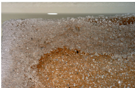
Figure 2: Illustration of efflorescence damages
